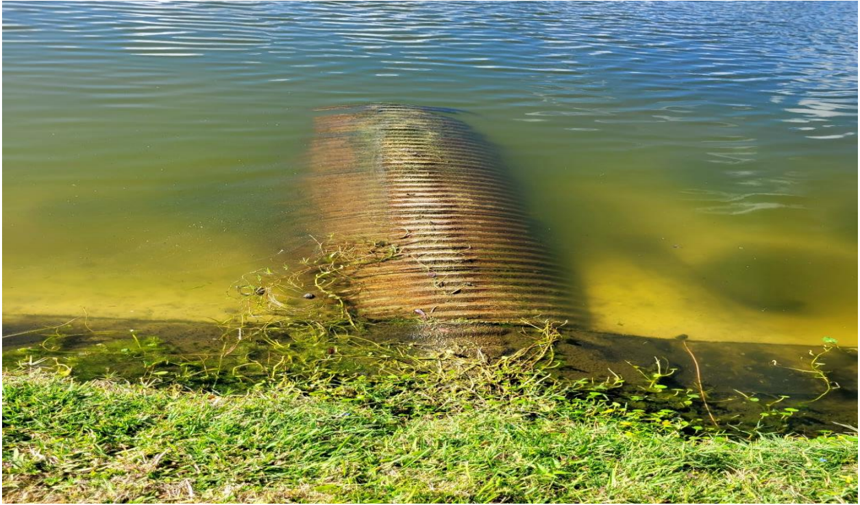
Photo 9: Corroded outfall pipe at Lake 4 (near NW 19 Court) during inspection in March, 2023.
