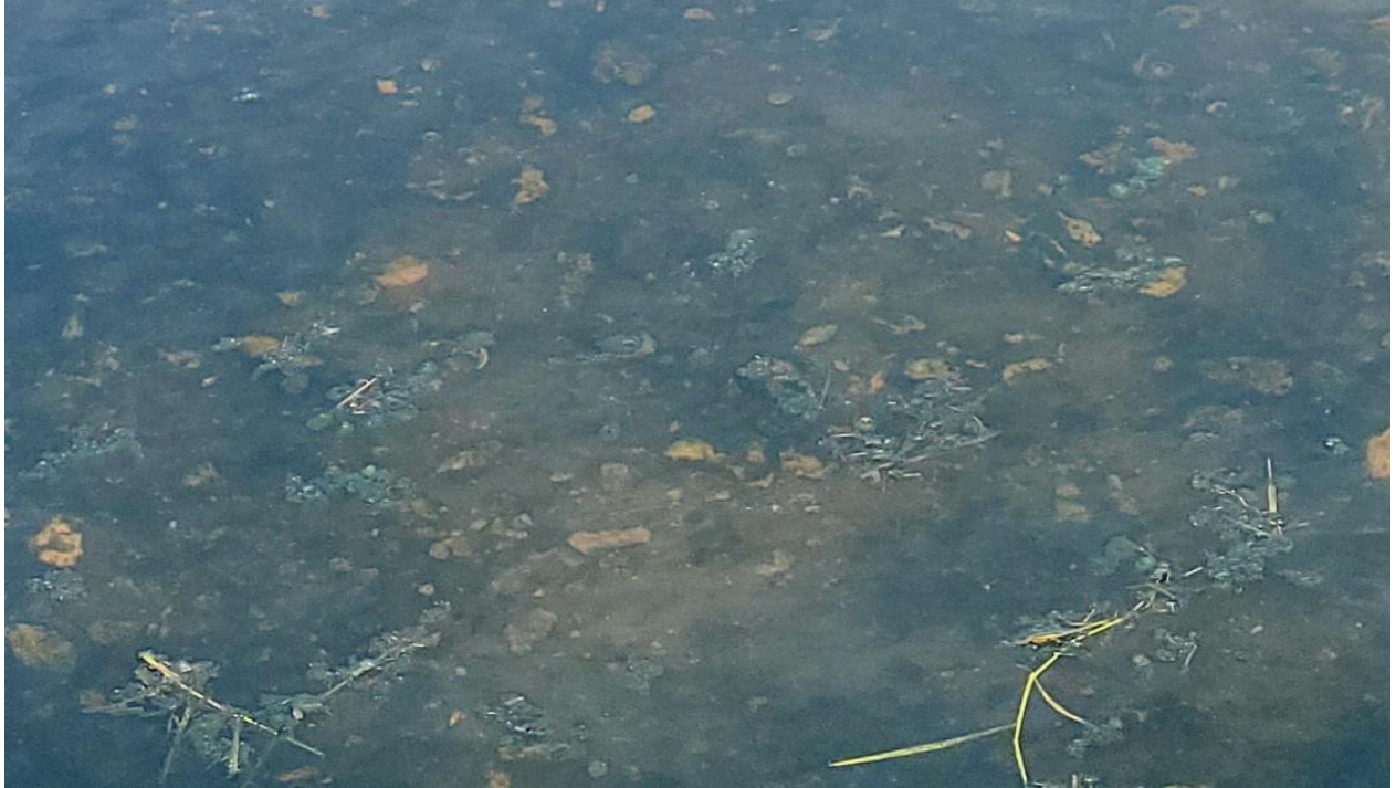
Photo 3: Depth of canal indicated as less than one foot due to bank erosion.
