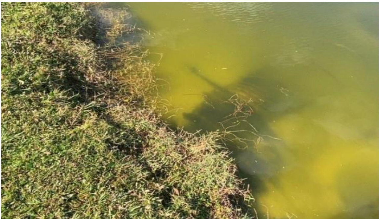
Photo 12: Disconnected outfall pipe extension at Lake 2 in June of 2024.
