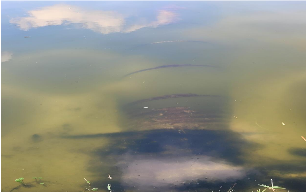
Photo 11: Corroded outfall pipe at Lake 4 during inspection in March, 2023.
