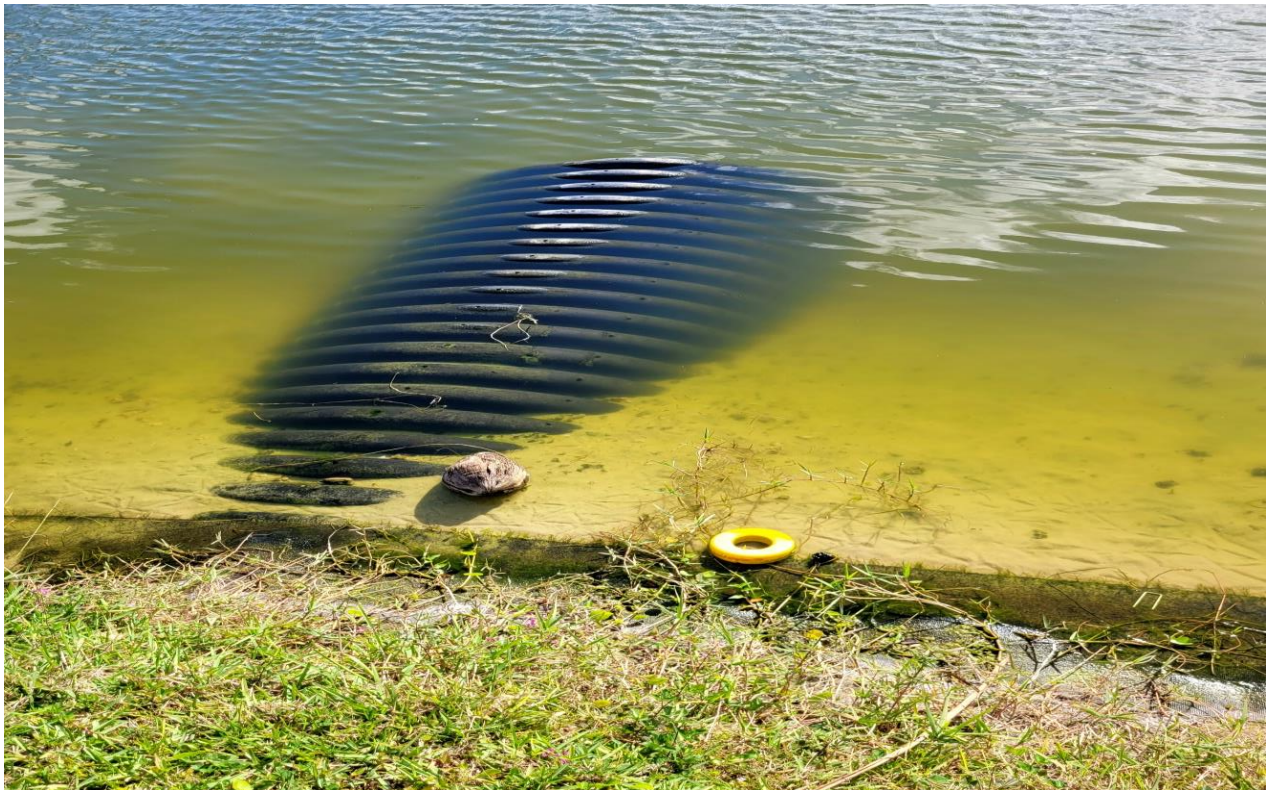
Photo 10: Sediment buildup at outfall pipe at NW 74 Ave in Lake 4 during inspection in March, 2023.
