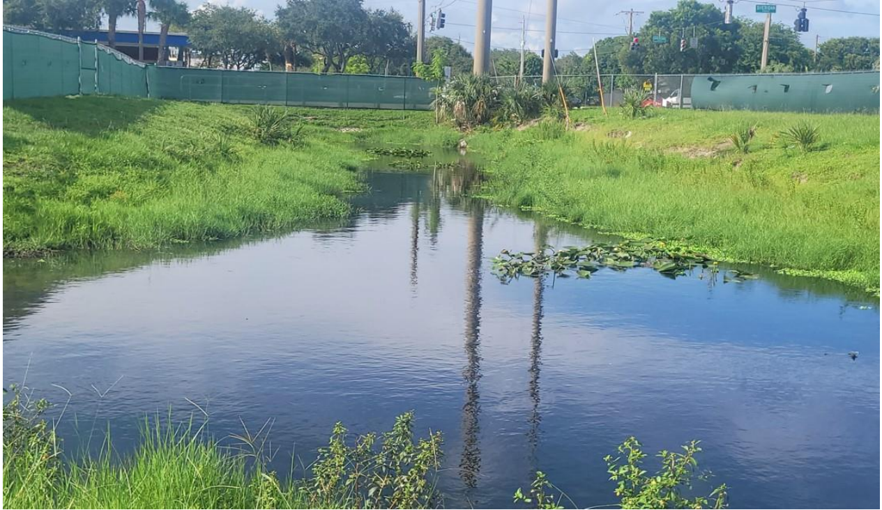
Photo 1: Canal bank erosion and capacity reduction at Sheridan Street and N 72 Avenue.
