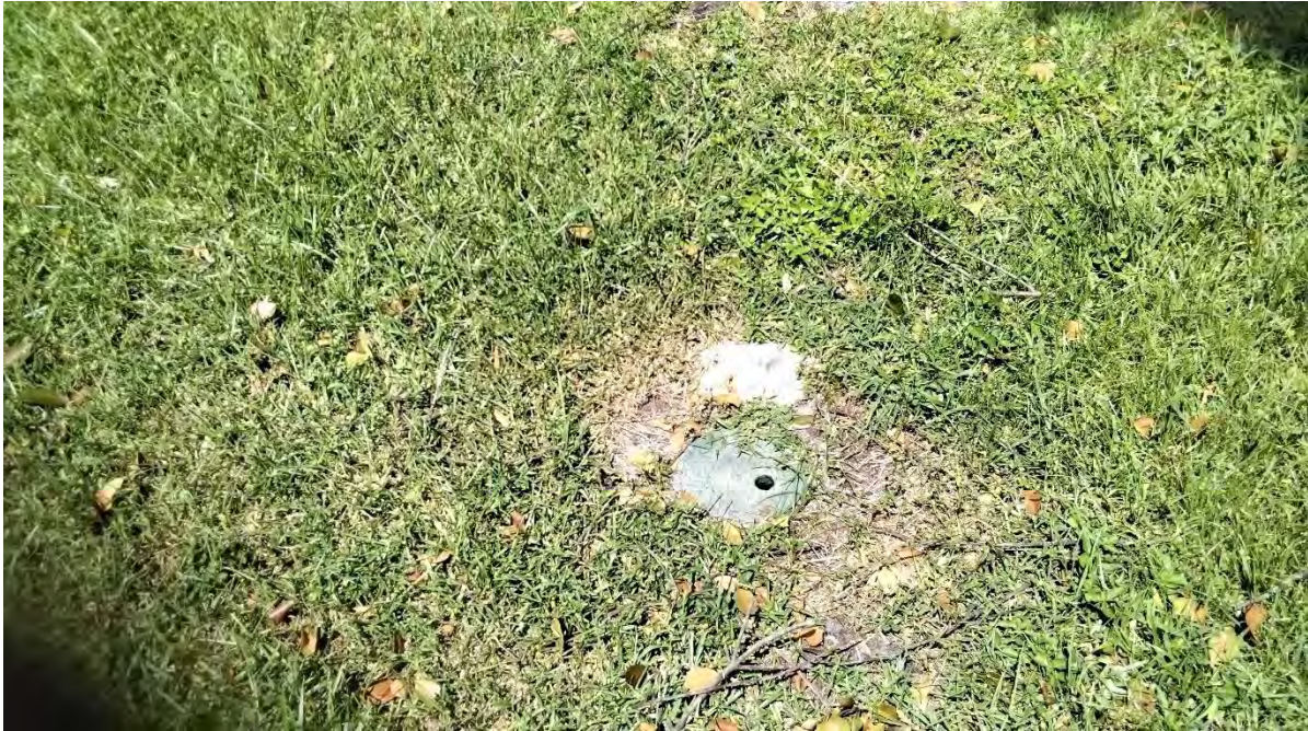
Above: Located along NW 20 th St. – An irrigation box has been overtaken by turf. Edging is required to assure location, maintenance and proper function.
