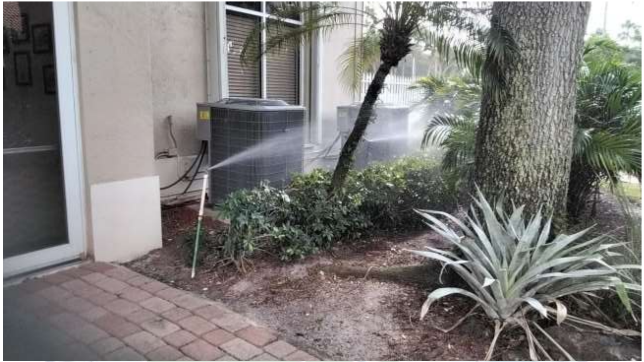
Above: Located along the perimeter of the Clubhouse – This is Zone 2 on the location clock. A riser is shown distributing water through a 45deg spray head and is well adjusted to the landscape bed. Pressure is good; however, one break was present and will be repaired.
