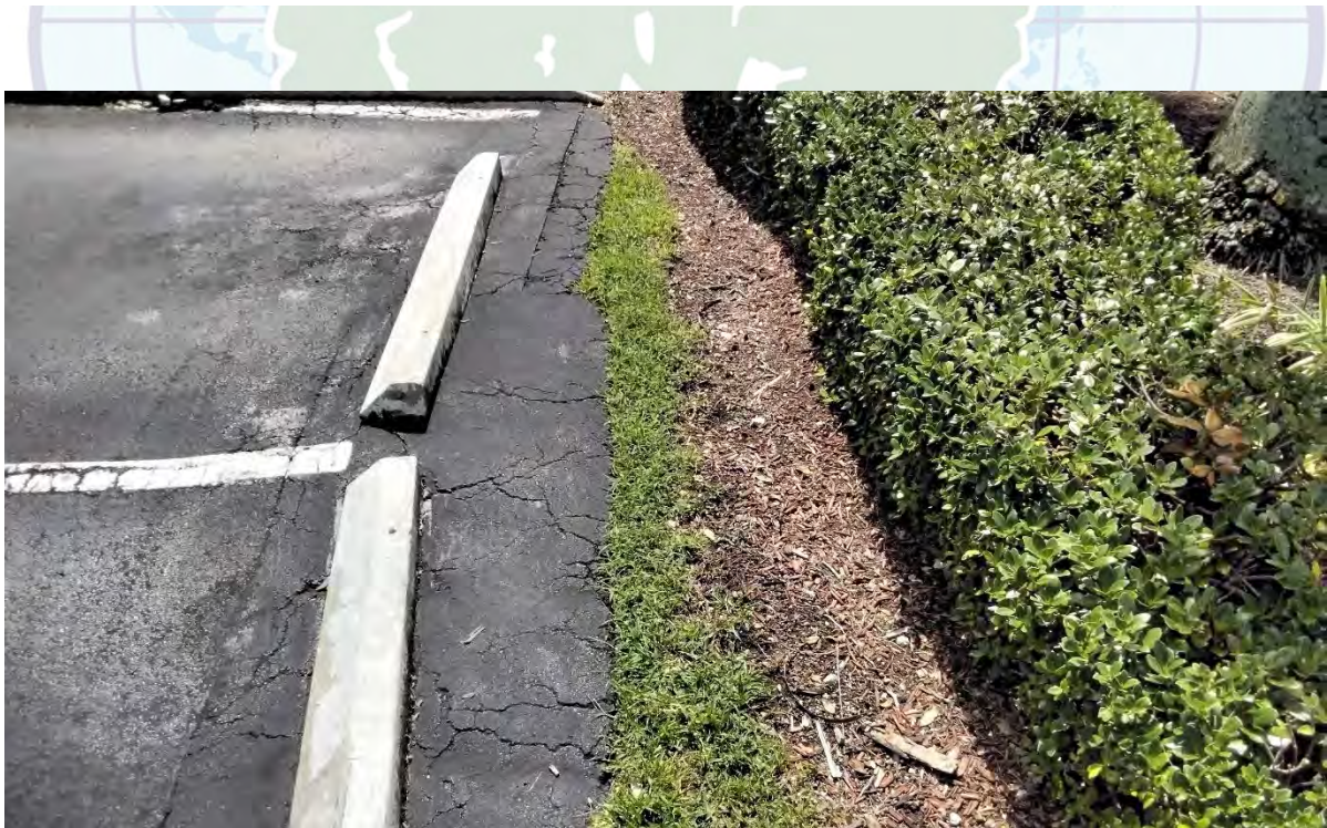
Above: Narrow strips of turf near parking areas and other hardscape are hard to maintain. Consider adding sod to widen the lawn to at least standard mower width (24" or wider), or remove these narrow strips and add mulch up to the hard surface. A border of perennial groundcover or dwarf shrubs as a second tier for these landscape beds is an enhancement to consider for community improvements.
