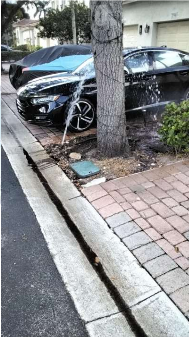
Above: Located near 7981 NW 20 th St - This is Zone 4 (a residential Zone) on the location clock. A broken head is shown. Tree root intrusion as well as pedestrian traffic/parking can be a continual cause of broken equipment.
