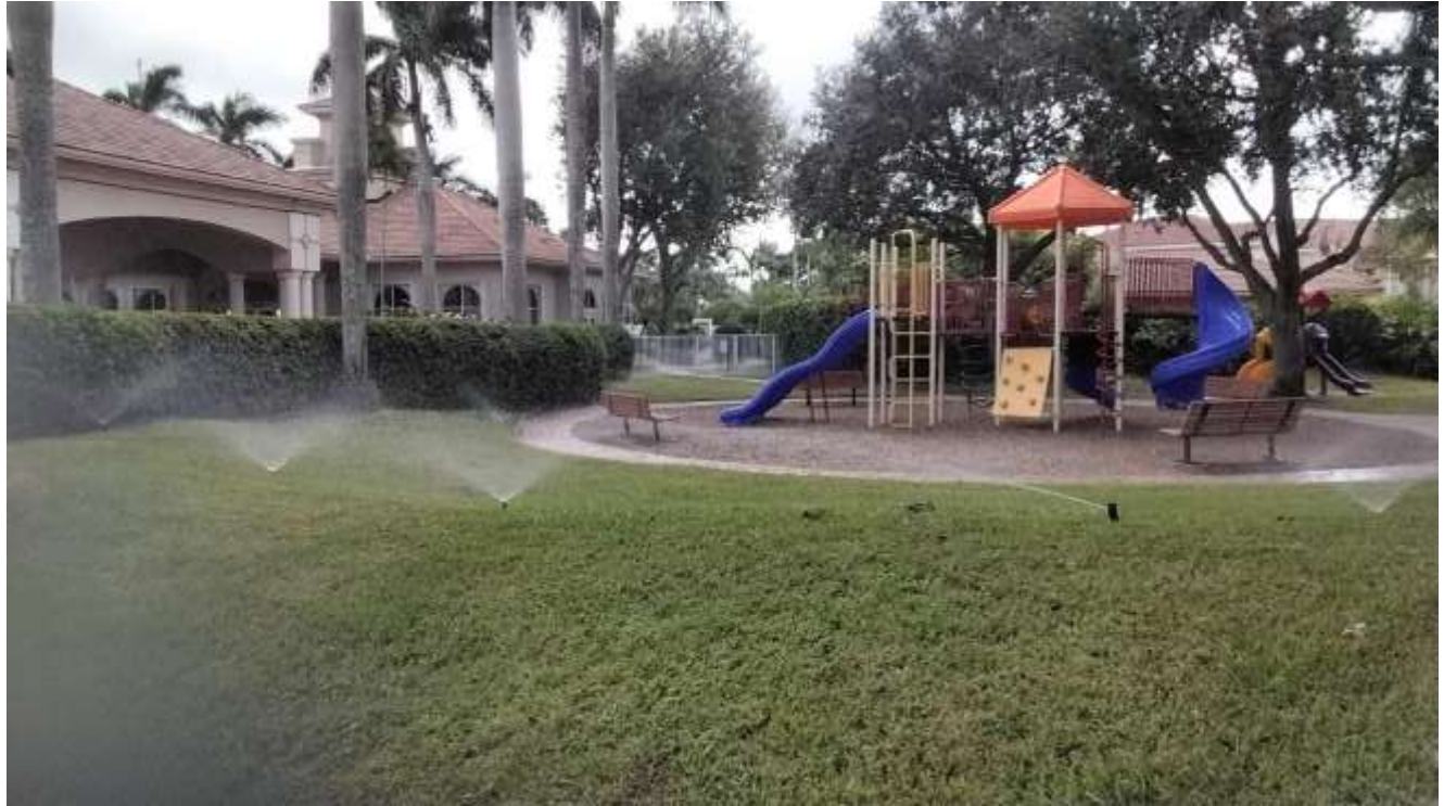
Above: Located at Clubhouse and Playground area – This is Zone 4 on the location clock. A mix of Rotors and Pop-up heads are utilized well here. There are some elevation changes and slopes here. Turf was consistent from high to low areas. Adequate pressure and coverage were observed.
