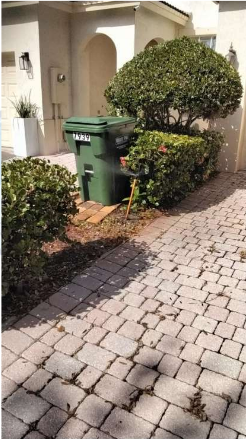
Above: Located near 7935 NW 20 th St. A residential irrigation zone is shown. Mostly Risers and Pop-ups are present. This is Zone 2 on the location clock. There is some adjustment needed in these areas as risers are leaning and some irrigation valve boxes need edging. Pressure is adequate in this location.
