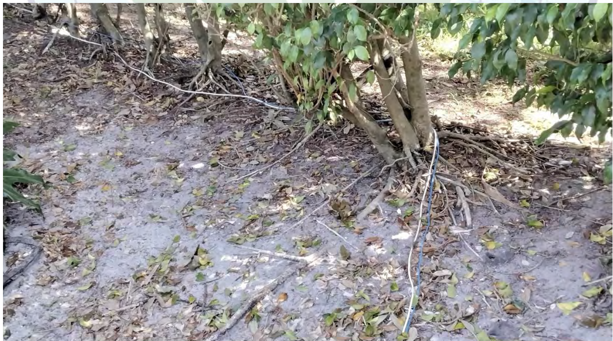
Above: Wires are shown running above ground and within the perimeter hedge. These wires can cause conflict with maintenance operations.
