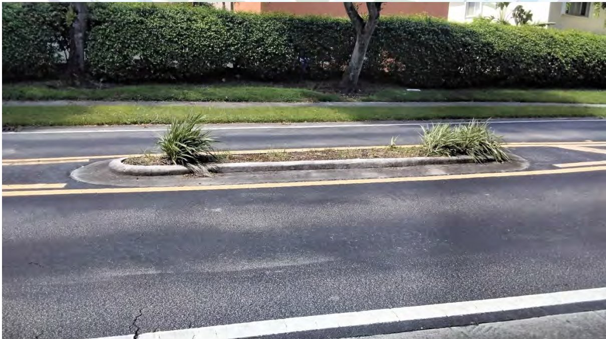
Above: A center median on NW 76 th St near the guard house is showing poorly. Missing plants, and excessive weeds are observed.
