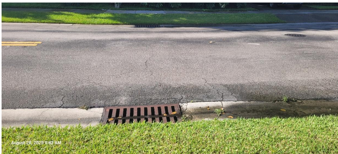
Photo 2: Depression and cracking of roadway and valley gutter above existing drainage pipe; caused by settlement.
