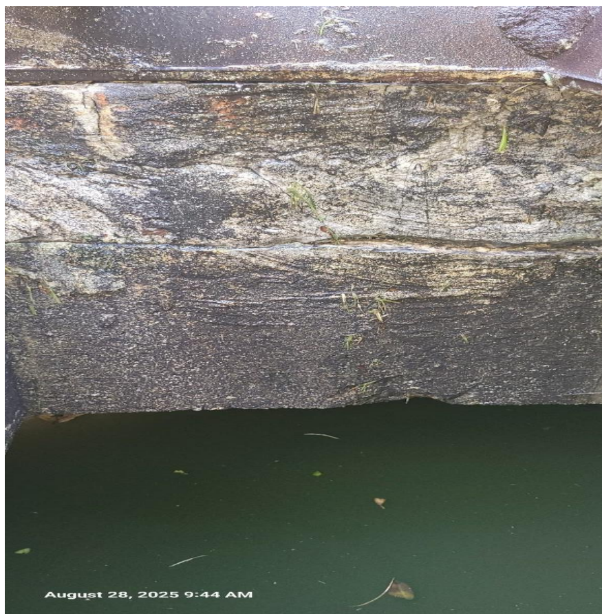
Photo 3: Minor cracking in catch basin 28. This picture is taken inside the catch basin, looking west toward the depressed area.
